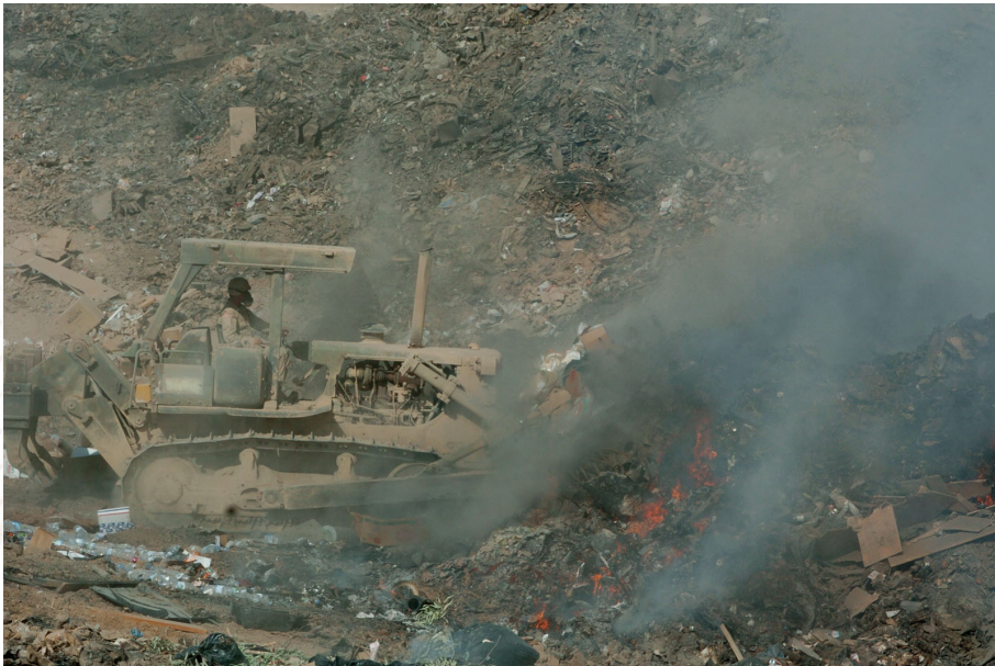
Sgt. Richard Ganske, 84th Combat Engineer Battalion uses a bulldozer to maneuver refuse into the burn pit.
